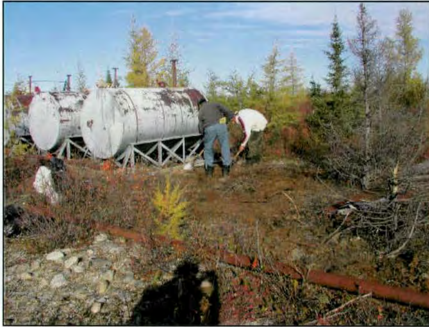
Photo 2 Application of the biological degradation process next to the fuel tanks at site 327A (27 September 2002).
